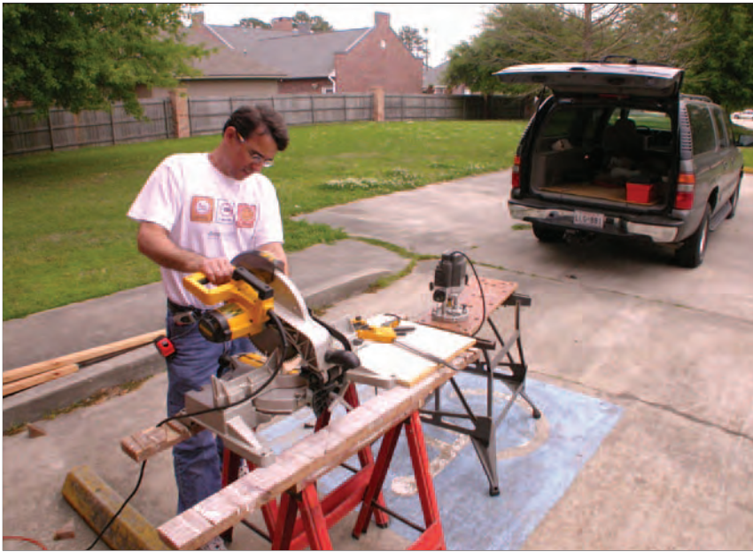
During the renovation, Allain tapped his experience building furniture to perform some of the finish carpentry himself.
